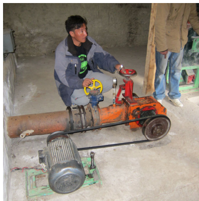
Servicing the Halji micro hydro system
